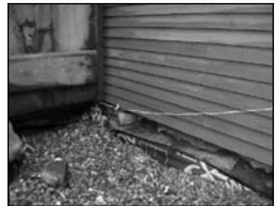
Water falling from the roof of the House into the French drain will be diverted away from the basement by the inclined barrier and stones.
