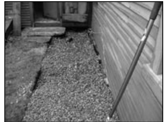
French drains were recently dug in two key areas around the House as a first step in relieving the humidity problems.
